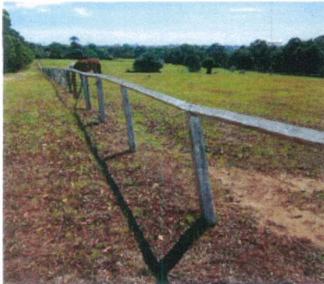
Private Road Fence (East) separating horses from the public road is in very poor condition.
